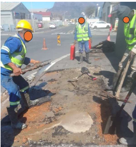
The CCT has been very busy this month working in Paarden Eiland to repair roads and other infrastructure.
